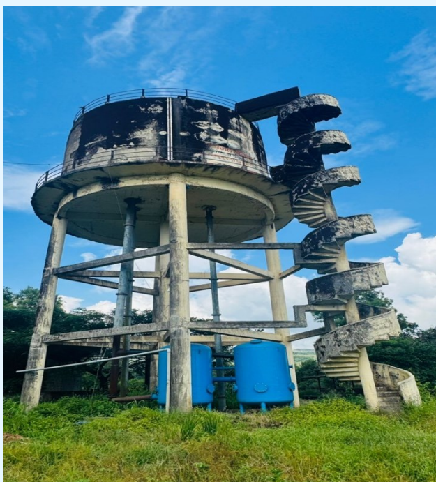
Overhead Tank at Gram Panchayat
