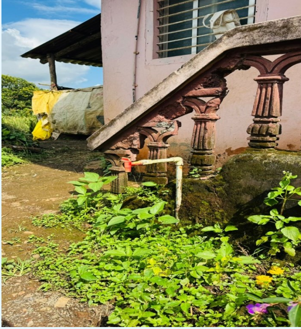
Pipeline Water Supply to Households
