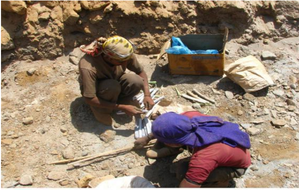
Laborers engaged in blasting activity for the 113-MW Andhra Lake Wind Power Project located at a distance of 3.5 km from the Bhimashankar Wildlife Sanctuary in Maharashtra
