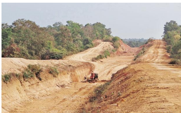
AN IRRIGATION CANAL UNDER CONSTRUCTION RUNNING THROUGH FORESTS IN BRAHMAPUTRA FOREST DIVISION ADJACENT TO TADоба TIGER RESERVE.
